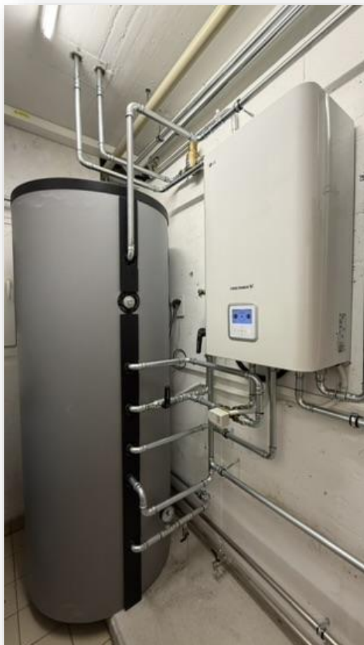
Boiler e centralina
